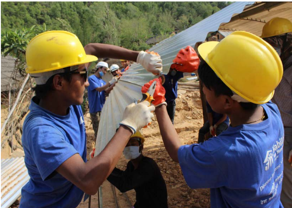
Volunteers join Habitat's rubble removal activity and construction of transitional shelters for families in Pipaltar, Panchkal, Kavre district on 2 June 2015.
